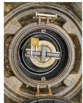
Closed fill port in a spill bucket
