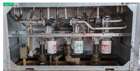
Under dispenser containment
