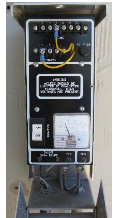
Rectifier, part of an impressed current system
