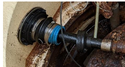
Test boot pulled back from wall of containment sump
