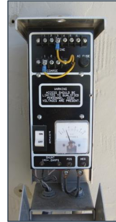
Example of a rectifier, which is part of an impressed current cathodic protection system
