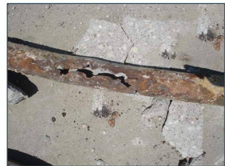
Example of corroded piping
