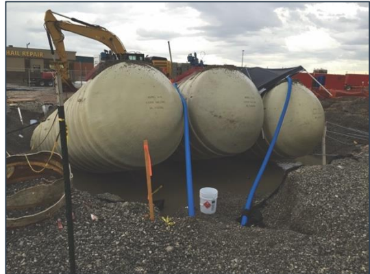
Tanks floating due to stormwater intrusion during installation before securing anchoring system
