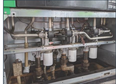
Inside of a dispenser cabinet
