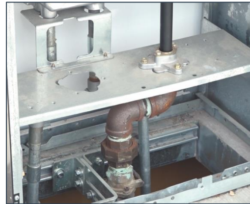
Example of a shear valve properly bracketed to concrete island
