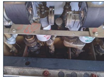
Example of under dispenser containment, or UDC
