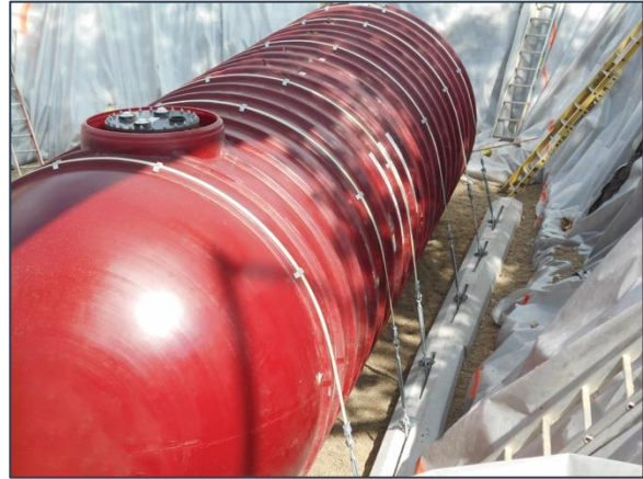
Tank being anchored to concrete deadman (right side, bottom of the basin) using straps
