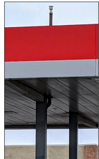
Example of vent line positioned above awning
