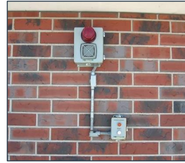
Example of an overfill alarm with attached emergency shutoff
