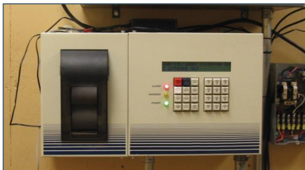
Example of an automatic tank gauge, or ATG
