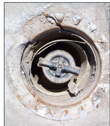
Example of a damaged spill bucket
