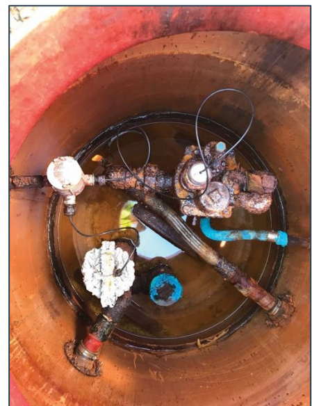
Example of corrosion due to bacterial growth (image courtesy of Ed Haselwood)
