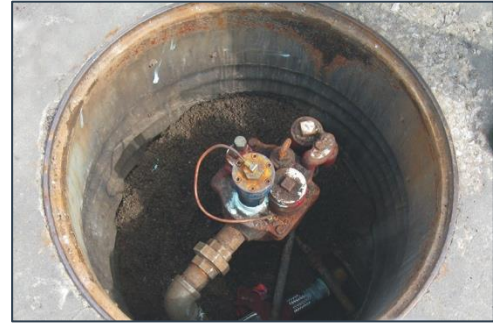
Example of an STP sump
