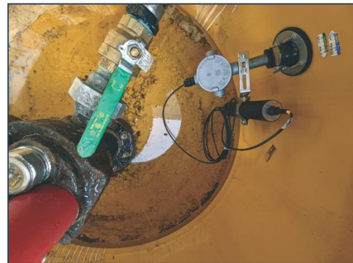
Example of a containment sump, which houses the pump and equipment related to release detection
